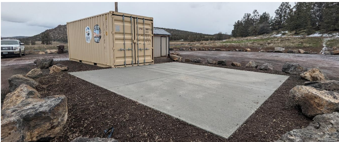
New concrete slab poured in February at the Barnes Butte Recreation Area for the use of a telescope.
