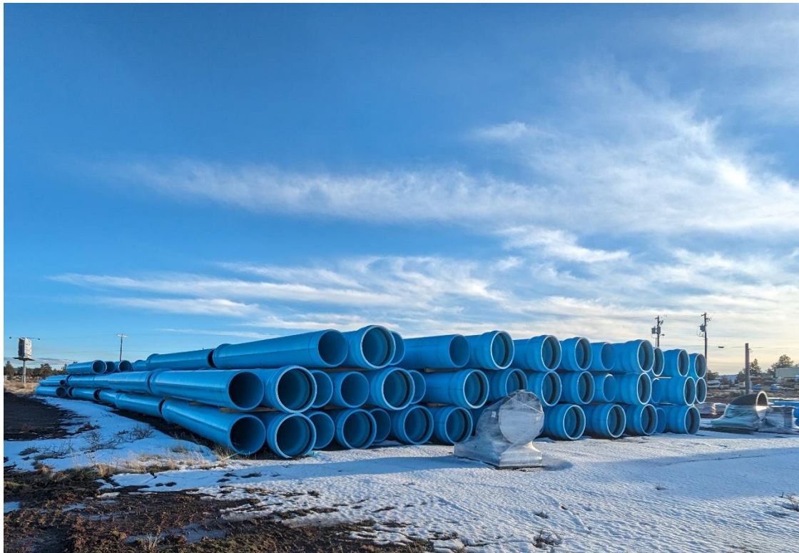
Pipe ready to be installed for the waterline extension project in the third quarter.
