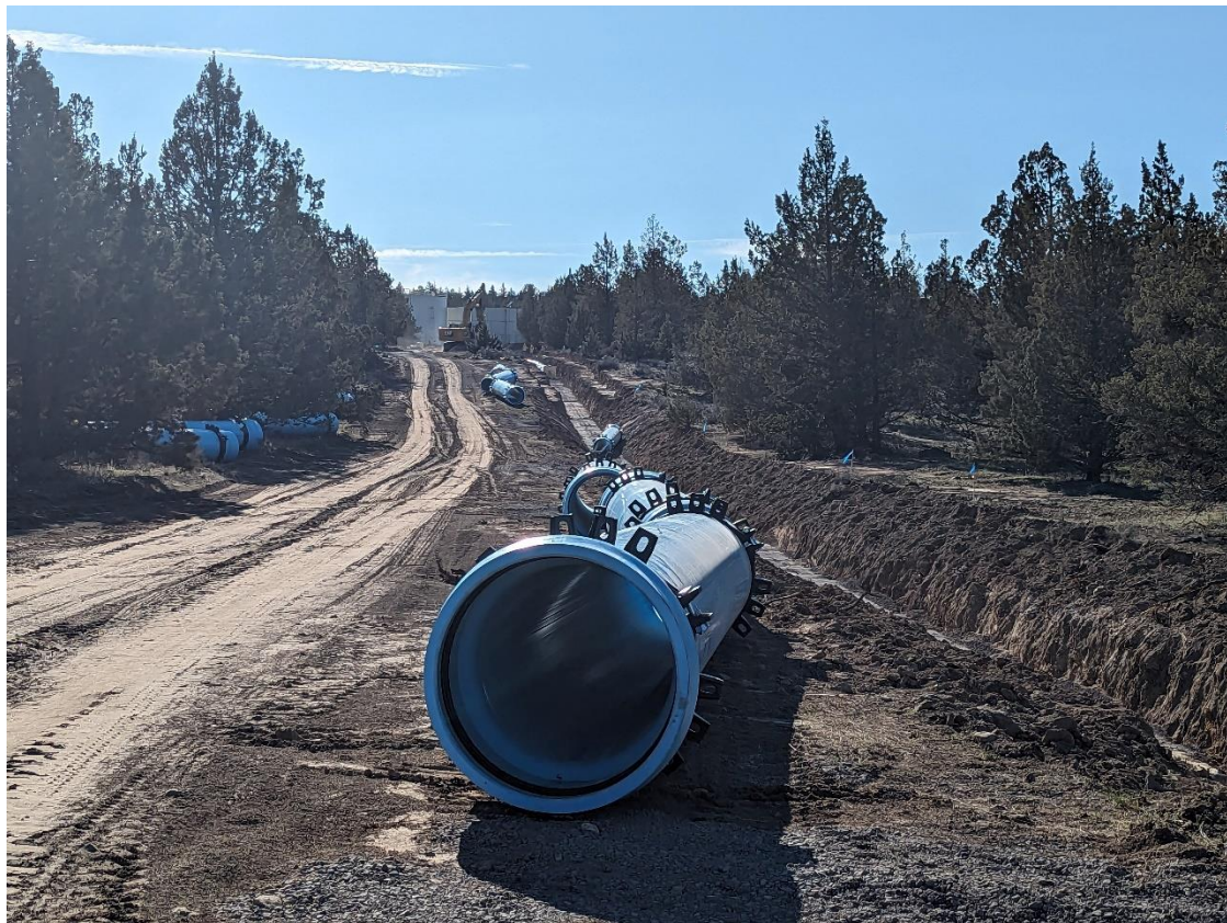
Pipe ready to be installed for the waterline extension project in the fourth quarter.
